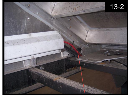
Use fish tape down side rail to pull 031-58992 RED 4GA 32' power wire into trailer nose.
